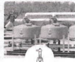
Filters, Dosing Pump & Injectors
